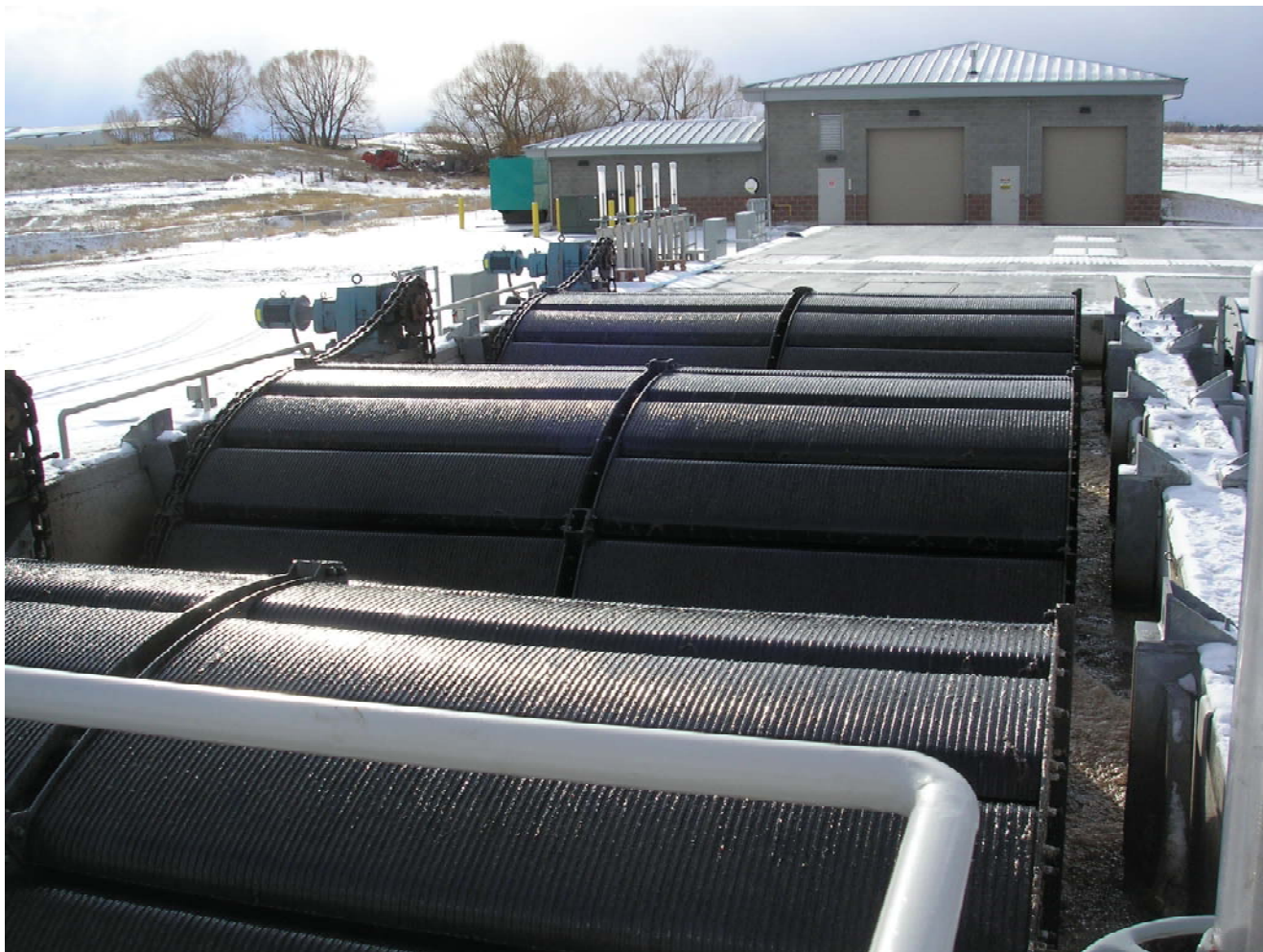
Figure 3D-4: Biowheel Installation at Manhattan Montana
